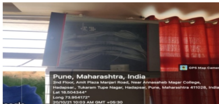
Chemistry 48 Port Switch
