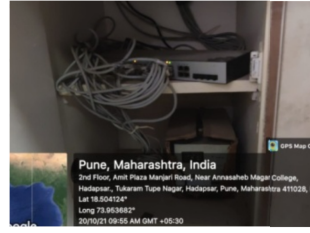
Electronics Department 48 Port Switch
