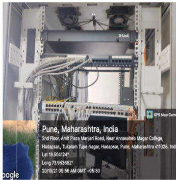
Main Service Port Switches
